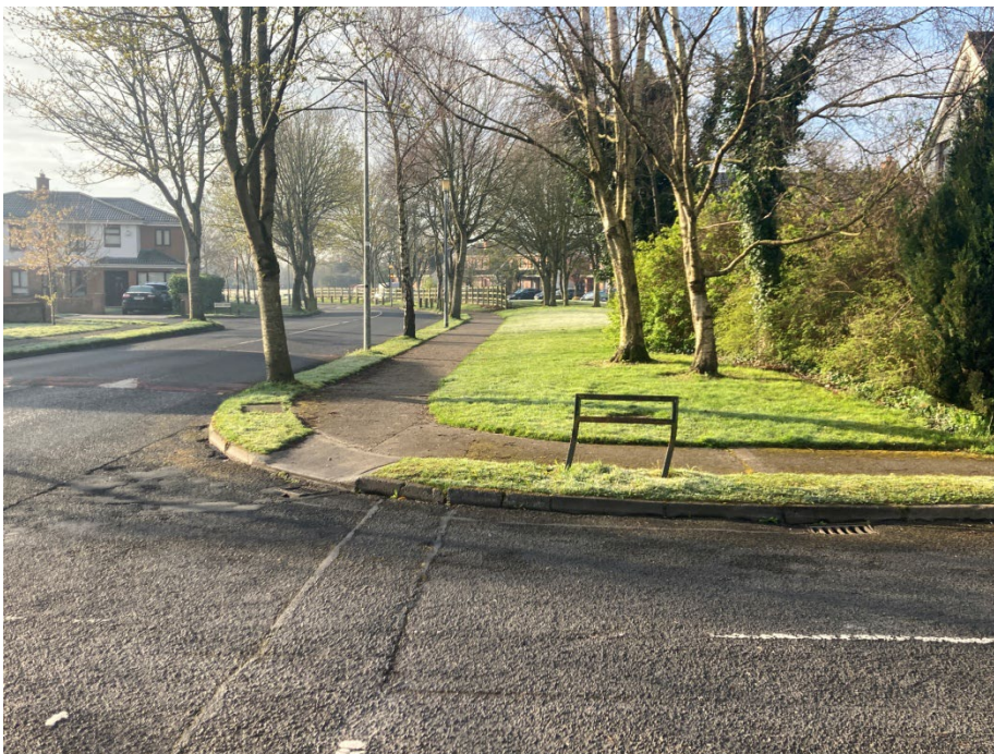
Image 5 – Damage Beaufield Close sign stand missing sign facing Newtown Road
