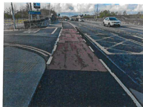
Straffan Rd – no kerbs + discontinued footpath
